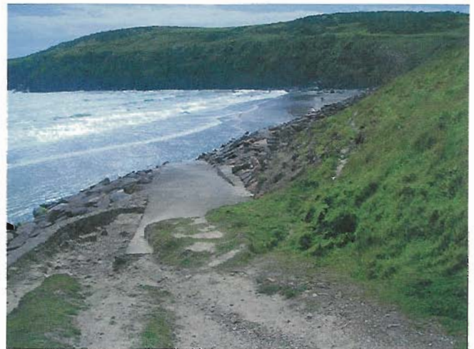
A small landslip has occurred
